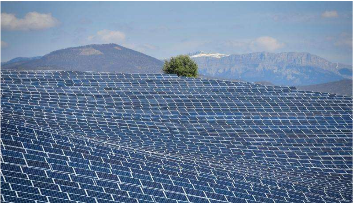
A solar farm at the Colle des Mees, in Provence.
